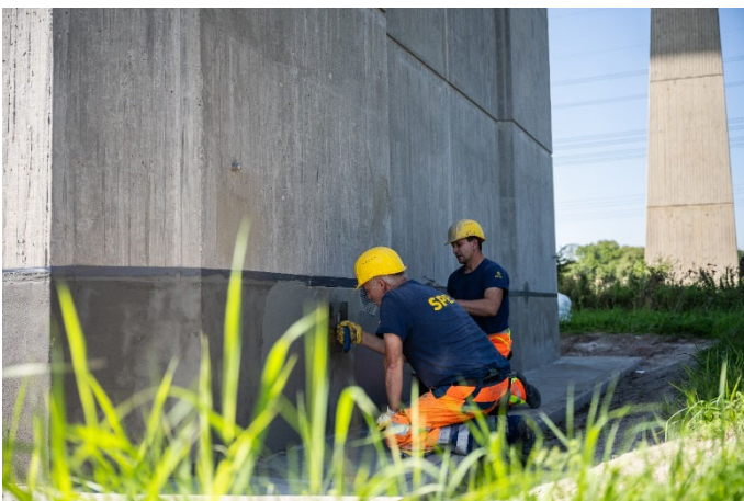
(5) To protect against penetrating moisture, the pier bases were also treated extensively.
