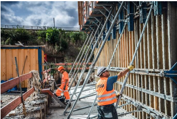
(4) The completion and commissioning of the new Aller bridge is planned for December 2024.
